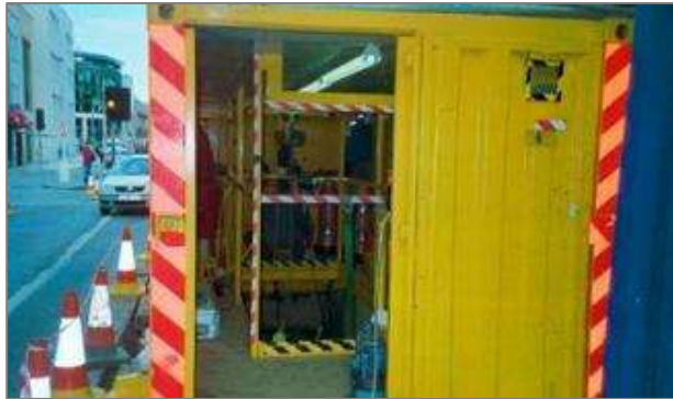
Figure 8.10: HV Cable Jointing Container
